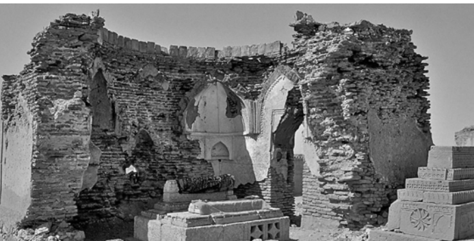
Restoration and Conservation Project, Stabilizing Endangered 15th Century Tomb of Samma Noble I, Makli Necropolis, Pakistan
